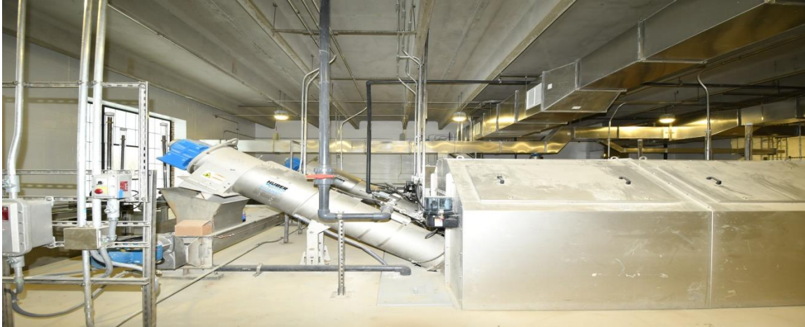
New Headworks Building upper level – fine screens
