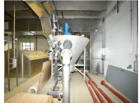
New grit removal system
