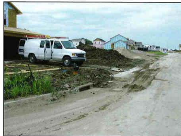
Lack of erosion and sediment controls during home construction threatens natural resources.
