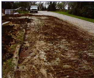
Without a proper entrance, sediment was tracked into the street and inlets carry sediment to the river.
