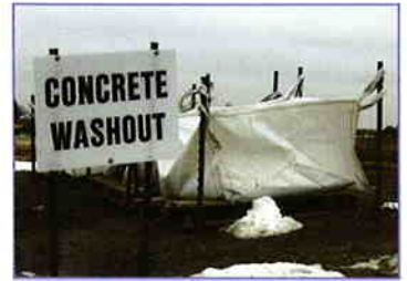
This designated concrete washout keeps pollutants from entering inlets and surface water.
